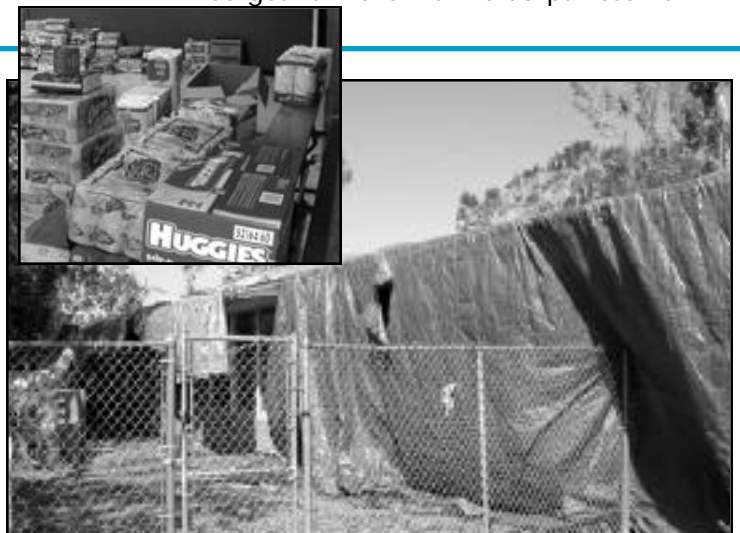
This was how Faith Lutheran School looked before the team of volunteers that Radetski was part of completed major structural repairs. Photo inset shows some of the truckloads of items that were donated to area residents.
